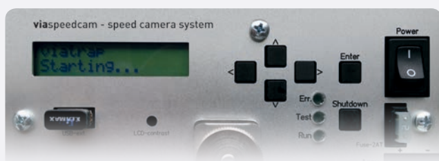
Control panel inside the battery box.
